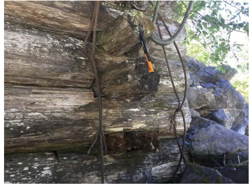
Left bank tie back condition - Poor
