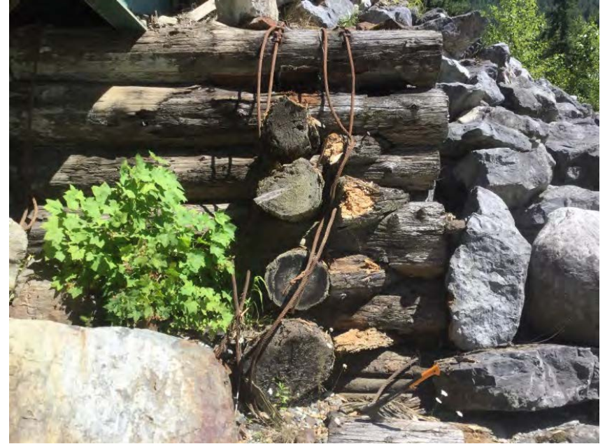
Right bank tieback condition - top upstream tieback sheared completely off, wing logs completely rotten at ends
