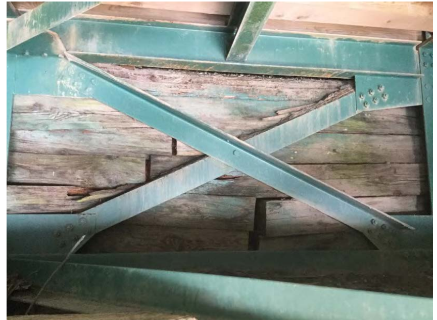
Right bank ballast wall - extensive rot
